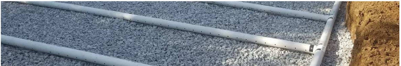
Below: perforated pipe is installed in a bed configuration with gravel beneath
